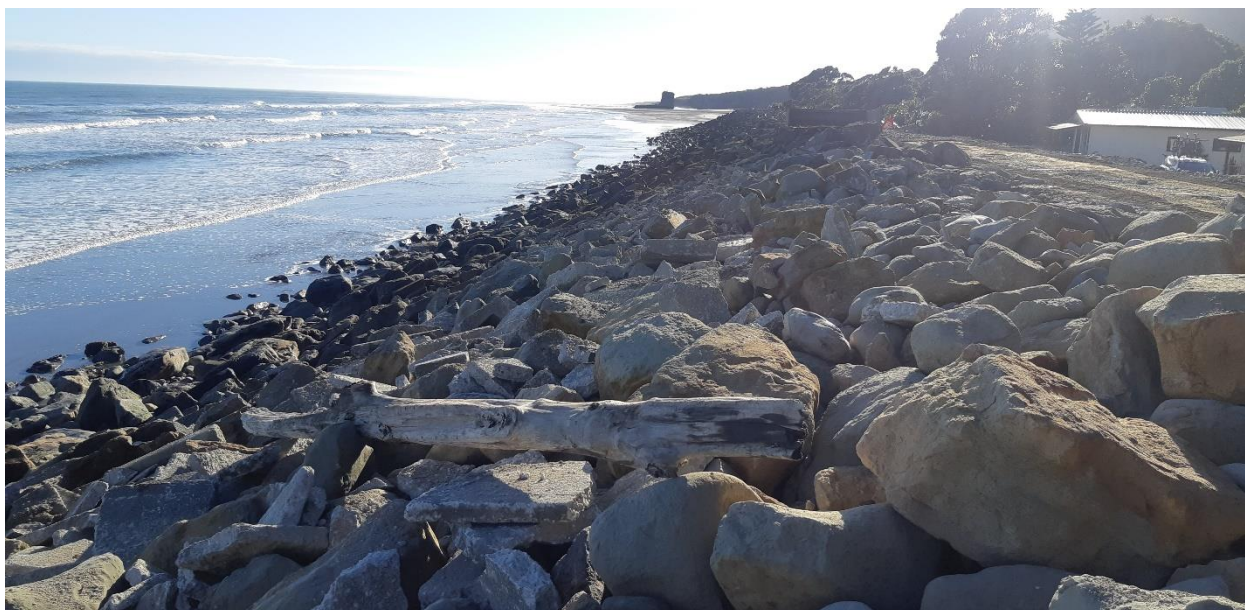
Punakaiki Seawall, looking North. Concrete sections interspaced between the rock armour on the front face of the revetment.
